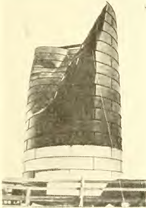
Failure of Metal Silo on Farm of E. W. Page, Goltry, Okla.
